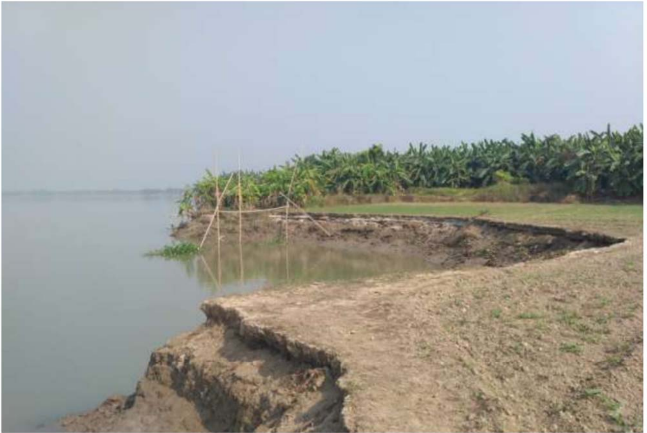
Plate 43 & 44 – Prominent bank erosion areas of Chakdah . 23° 3'9.44"N 88°27'28.23"E & 23° 3'33.89"N 88°27'28.56"E
